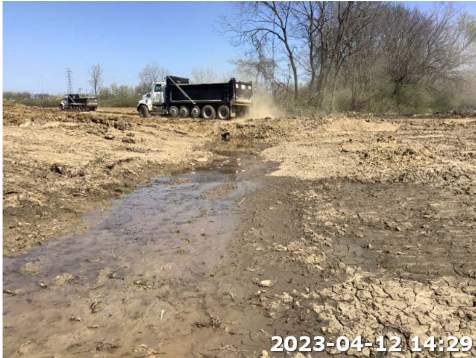
Photograph Location 23. Representative view of existing culvert and upland drainage feature. Photograph taken facing northeast.
